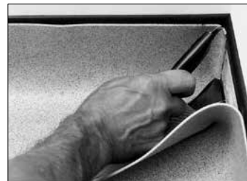
3. Fold in one side and gradually cut off the surplus FiberFlex® to complete the first part of the corner.
